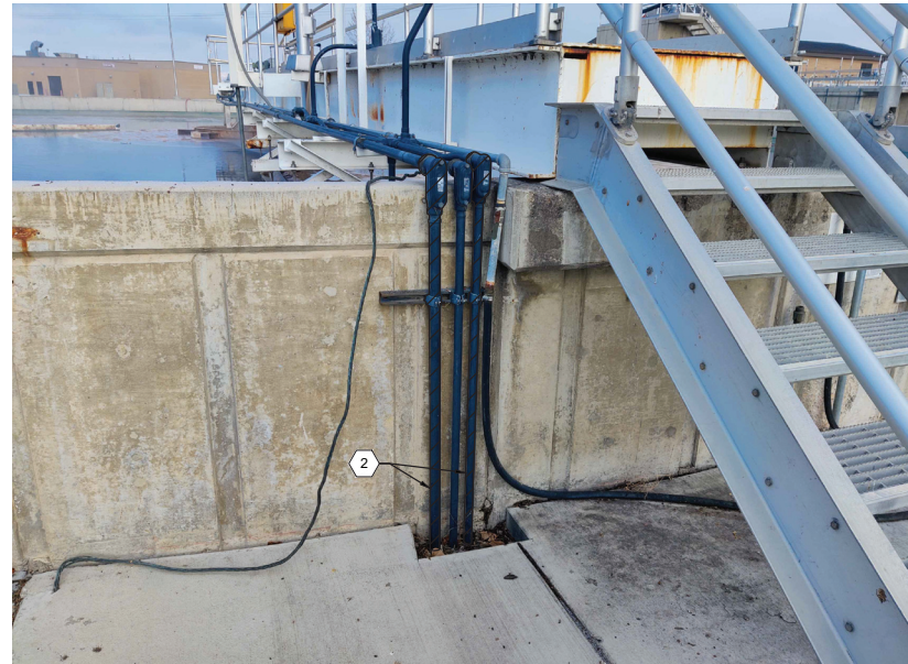
CLARIFIER E-1 VIEW NORTH CONDUITS SCALE: NTS
