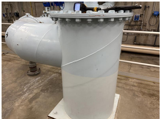
Photo #34 January 31, 2025: Filter gallery old side, two tone pipe –Lead concentration: White 0.47 mg/cm 2 , light blue 0.24 mg/cm 2
