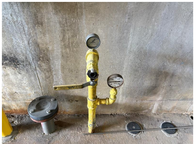
Photo #22 Chlorine loading dock valve—Lead concentration: 5.00 mg/cm 2
