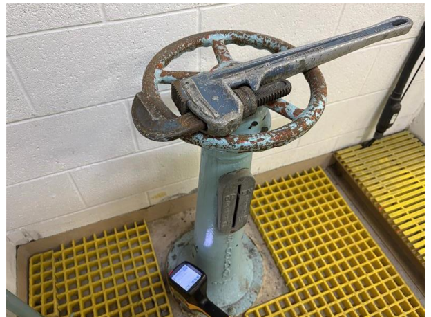
Photo #20 Chlorine room blue valve—Lead concentration: 1.00 mg/cm 2
