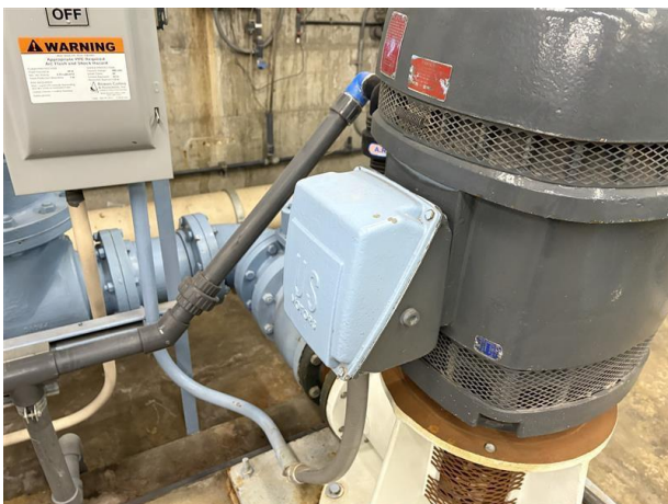
Photo #35 January 31, 2025: Filter Gallery old side, light blue electric cover on gray pump—Lead concentration: 0.32 mg/cm 2
