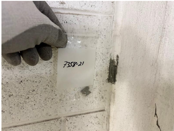
Photo #7 HA-07: Gap filler in Chlorine Room, not asbestos containing
