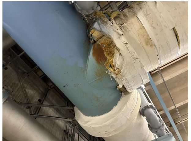
Photo #32 January 31, 2025: Filter Gallery old side, south side teal backwash header pipe running east-west—Lead concentration: 3.72 mg/cm 2
