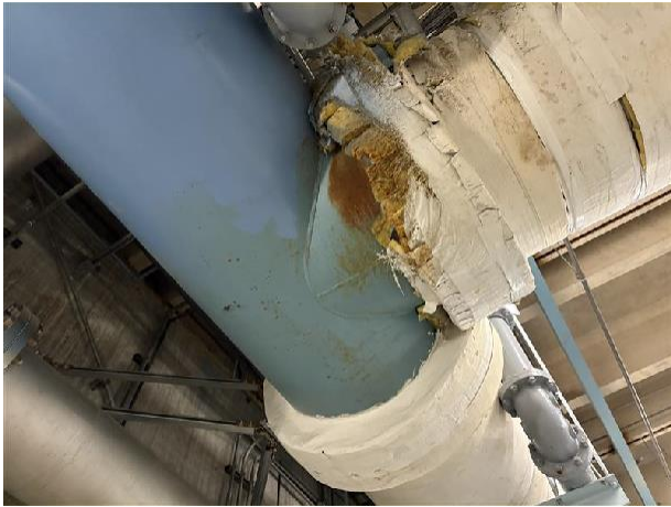
Photo #31 January 31, 2025: Filter Gallery old side, south side teal backwash header pipe running north-south—Lead concentration: 3.70 mg/cm 2
