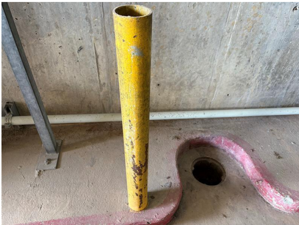
Photo #21 Chlorine loading dock bollard—Lead concentration: 5.00 mg/cm 2
