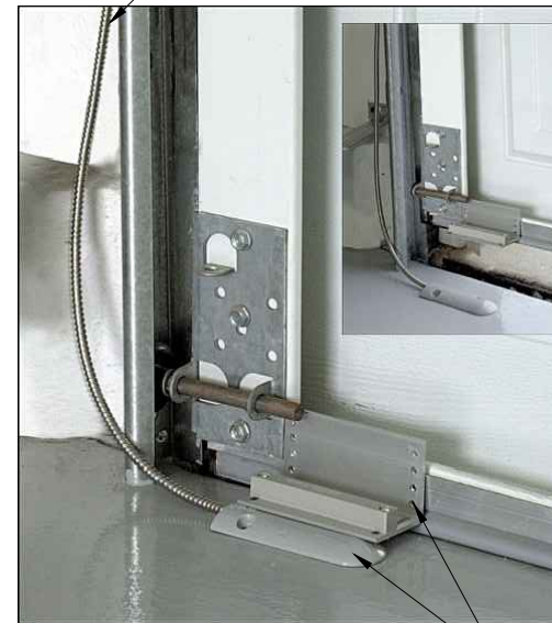
FLOOR MOUNTED SWITCH. MANUFACTURED BY GEORGE RISK INDUSTRIES, INC. MODEL 220-36 OR EQUAL
