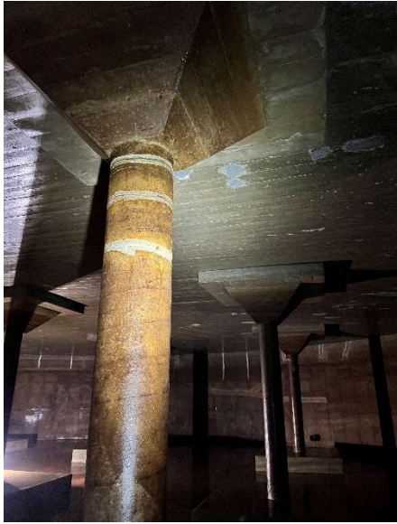
Wrapped column cracks
