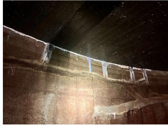
Patched cracks at roof joint
