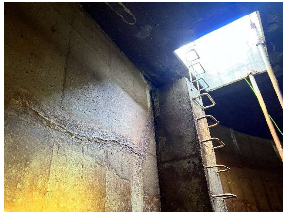
Overflow, valve stems, and access hatch
