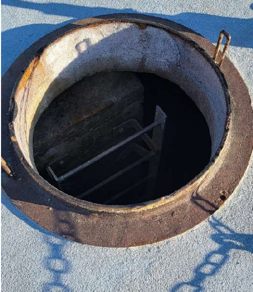
Access manway – broken seal
