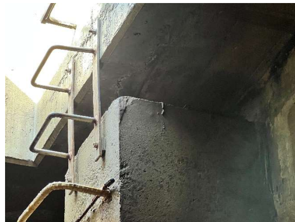
Top of overflow
