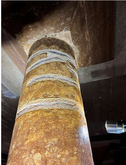
Wrapped column cracks
