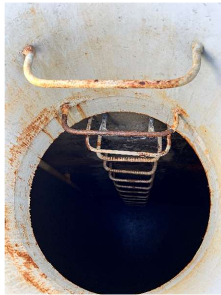
Manway looking in – rungs in need of recoat
