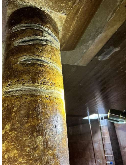
Wrapped column cracks
