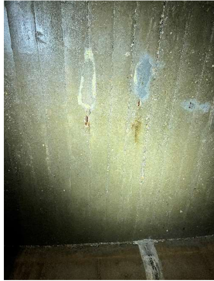
Roof spalling patches
