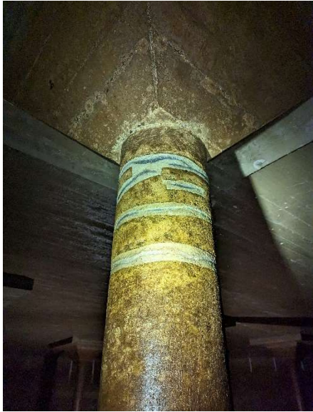
Wrapped columns cracks
