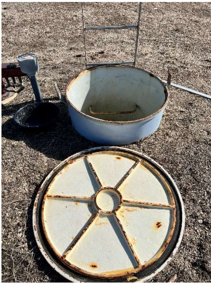
Manway – lid and ladder-up
