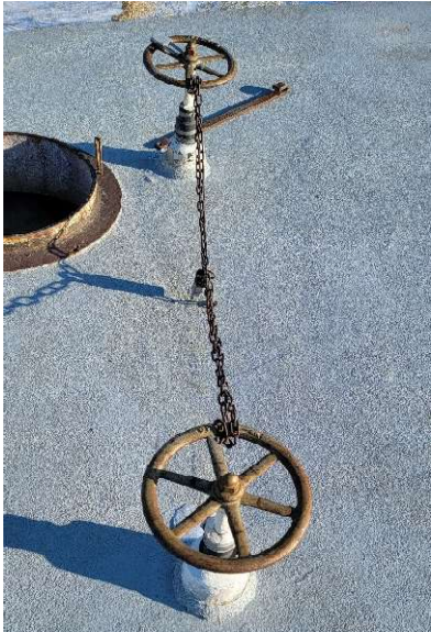
Valve actuators – locked
