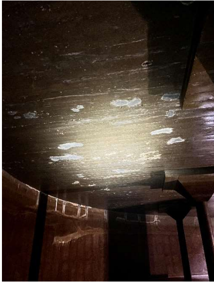
Roof spalling patches
