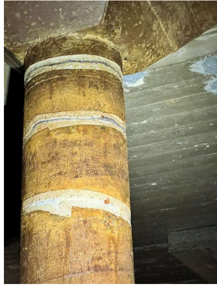
Wrapped column cracks
